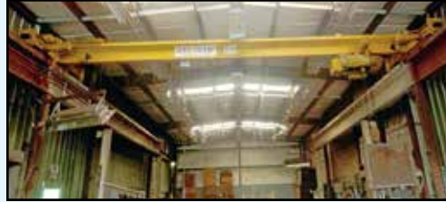
DIXIE Bridge Crane , 5-ton, Chandler Henry hoist, single-grinder, top running, under hung hoist, pendant control.
