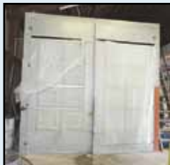
Paint Booth, 12' x 24', explosion proof lights.
